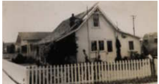
Daddy working on the roof of our San Diego home about 1946. Notice our trailer parked in back - guess they were keeping a way back to Ohio, just in case.
